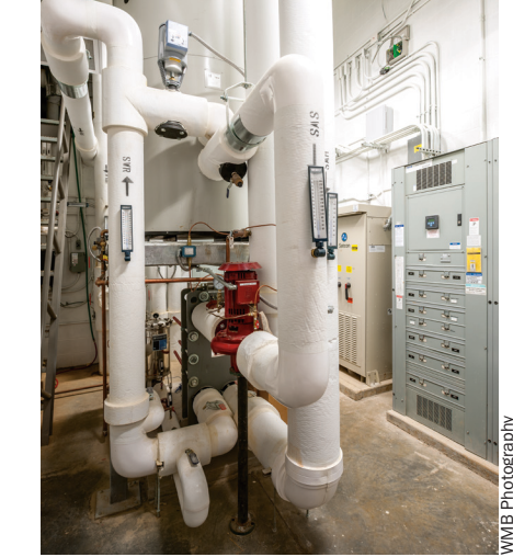
The solar thermal panels heating the domestic water have an electric heating element for backup.
